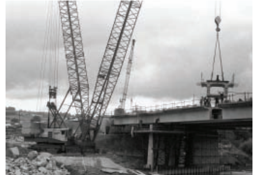
Greg Perks' experience of bridge building includes construction of an early glued segmental balanced cantilever on the Brecon Bypass – here in 1980
