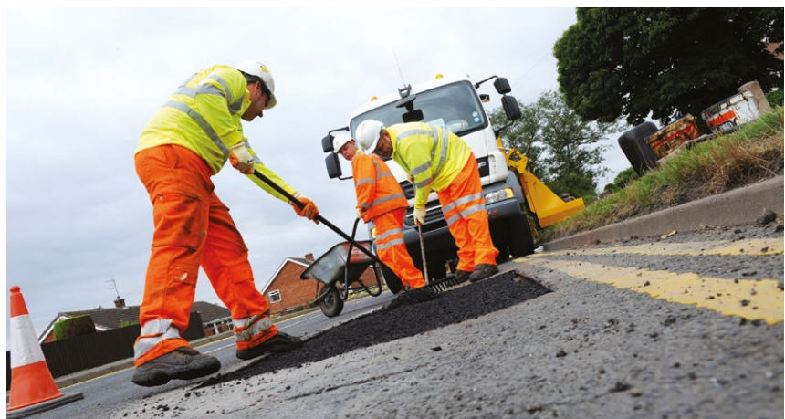
Highway maintenance is covered by the UKRLG's newly revised Codes of Practice
