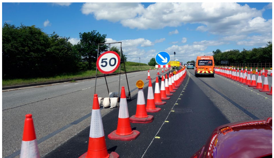
↑ Highways England is working to reduce driver frustration through temporary works ALASTAIR LLOYD
