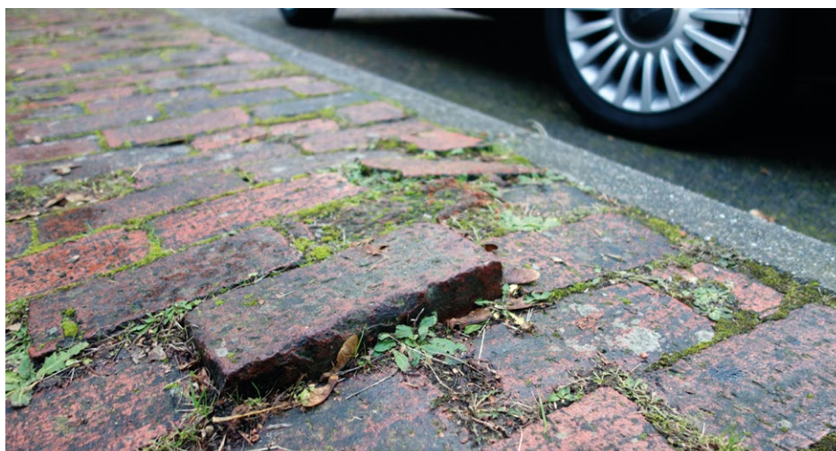
↑ Damaged footways present both a trip hazard for pedestrians and a financial liability for authorities
