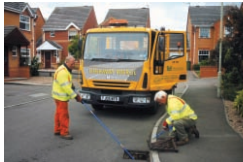
Asset management: great breadth and depth of work is involved applying the approach to every road asset
