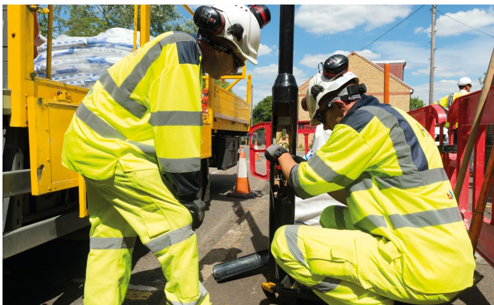
↑ Street lighting in Hounslow now features LED luminaires RINGWAY HOUNSLOW HIGHWAYS
