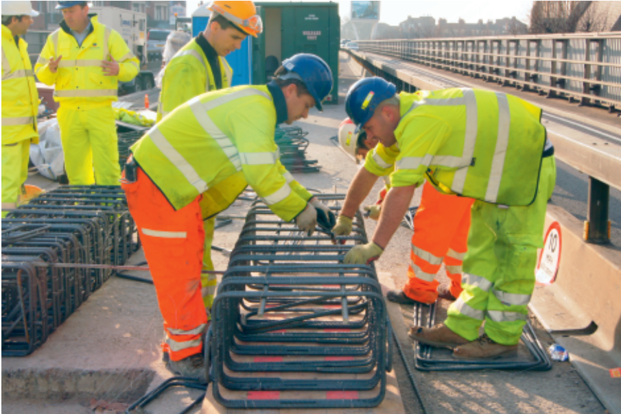
Local authorities now have extra help in implementing asset management with new guidance
