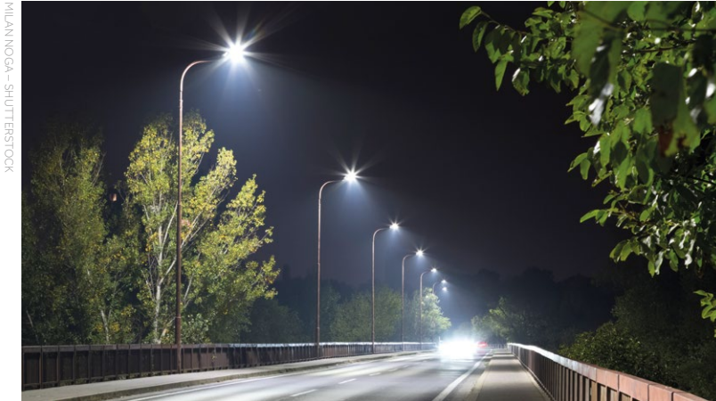
↑ Huge financial savings can be realised from installing the latest lighting
